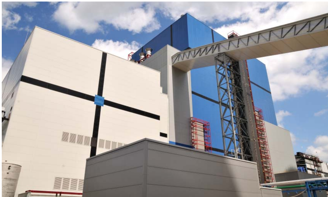
Foster Wheeler 460 MWe, gross boiler in Lagisza, Poland. World's largest and first supercritical once-through CFB boiler.
