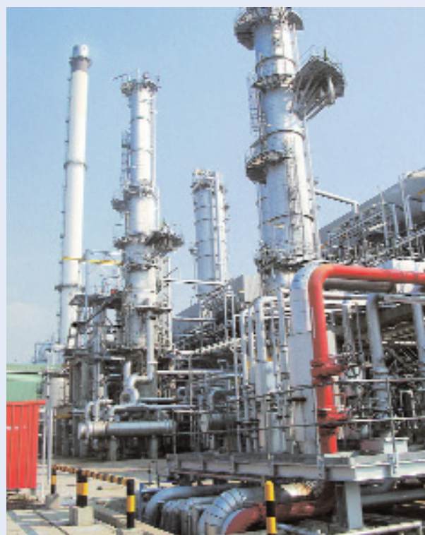
View from north-west corner of process units, including Parex™ unit finishing column (foreground), and the 140-metre reinforced concrete stack (background).
