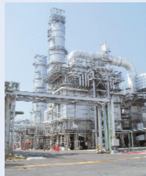
Process units from south-east - xylene rerun column with its reboiler heater.
