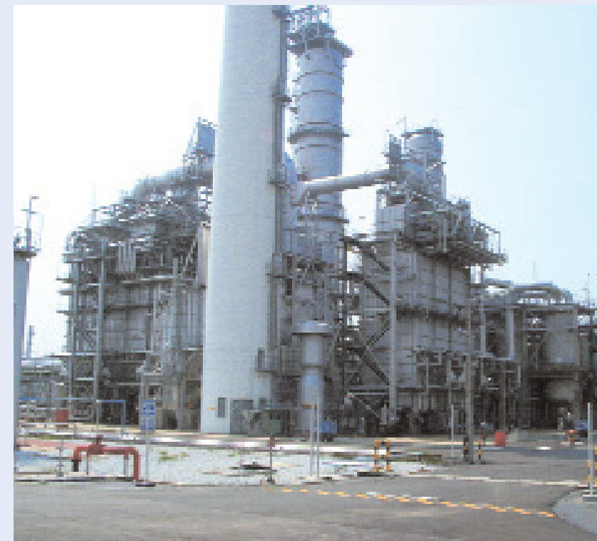
View of process units from north-east - fired heaters with their associated concrete stack.
